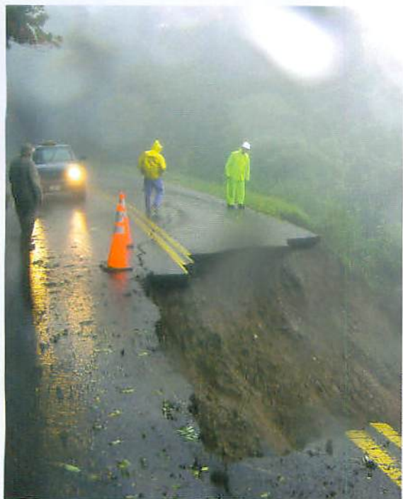
Milepost 348.6. Officials inspect the unprecedented damage of more than a full lane being washed away.
